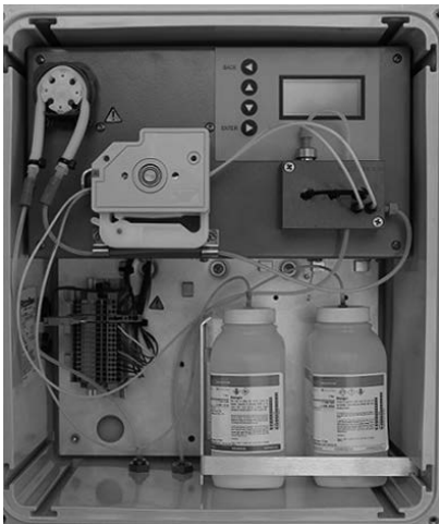
Figure 6: Sample pump shown with cover off
